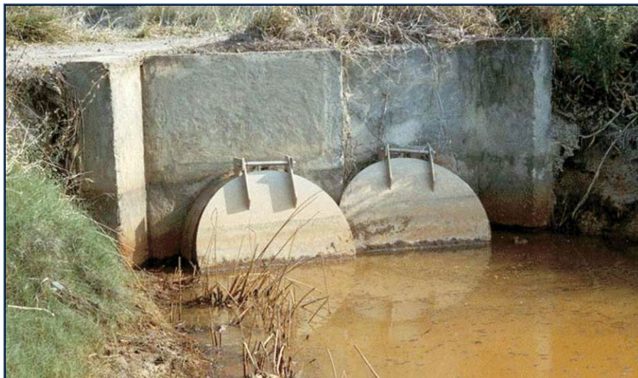
Figure 4. Iron scum smothers vegetation and coats structures.
