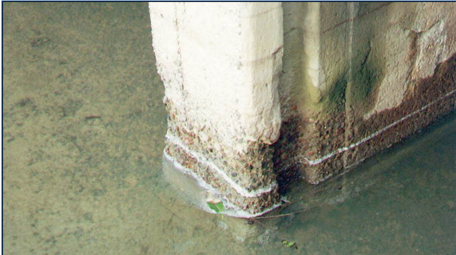
Figure 5. Degradation of concrete by acid water.
