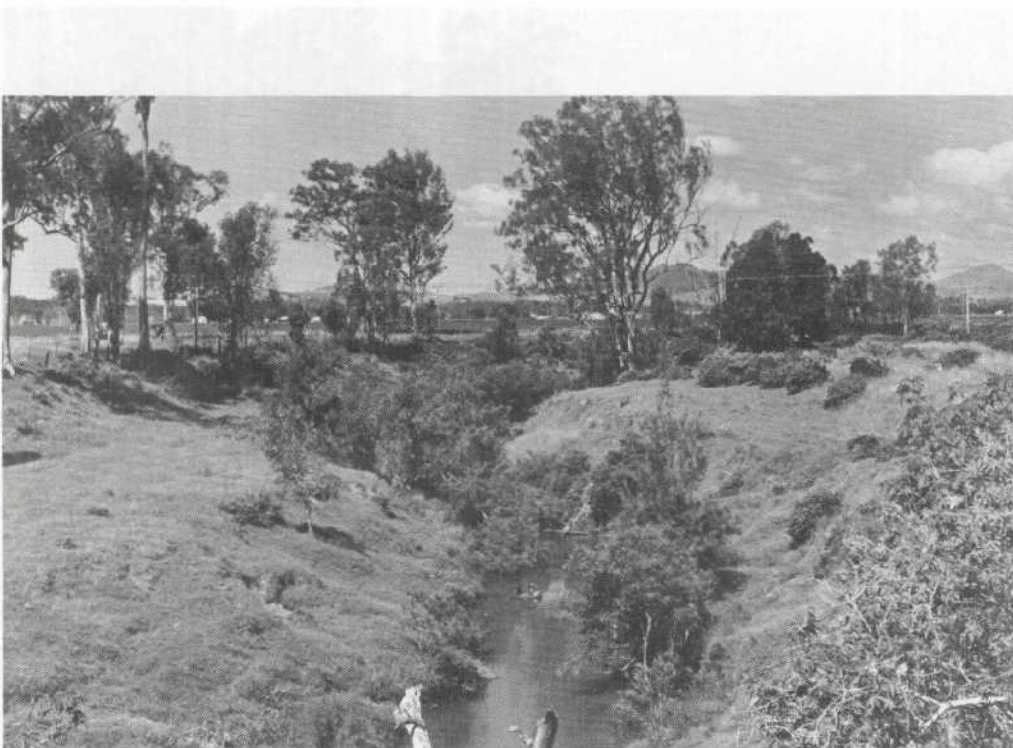
Creeks crossing the alluvial plains have deeply incised channels, but are rapidly becoming choked with vegetation and silt.
