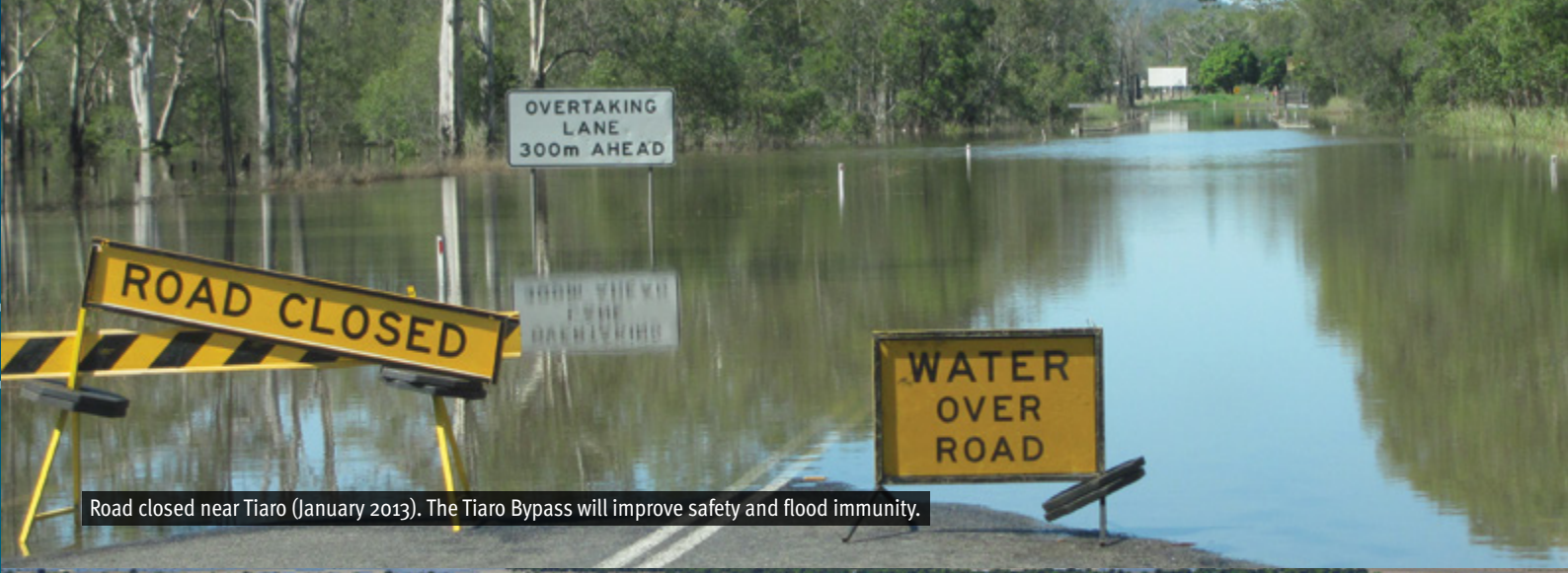
Caboolture-Bribie Island Road to Steve Irwin Way (Exit 163), bridge works at King Johns Creek (August 2021).
