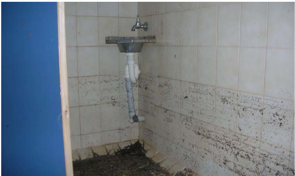
Photo 36. Inundation water levels within a public toilet block at Wongaling.
