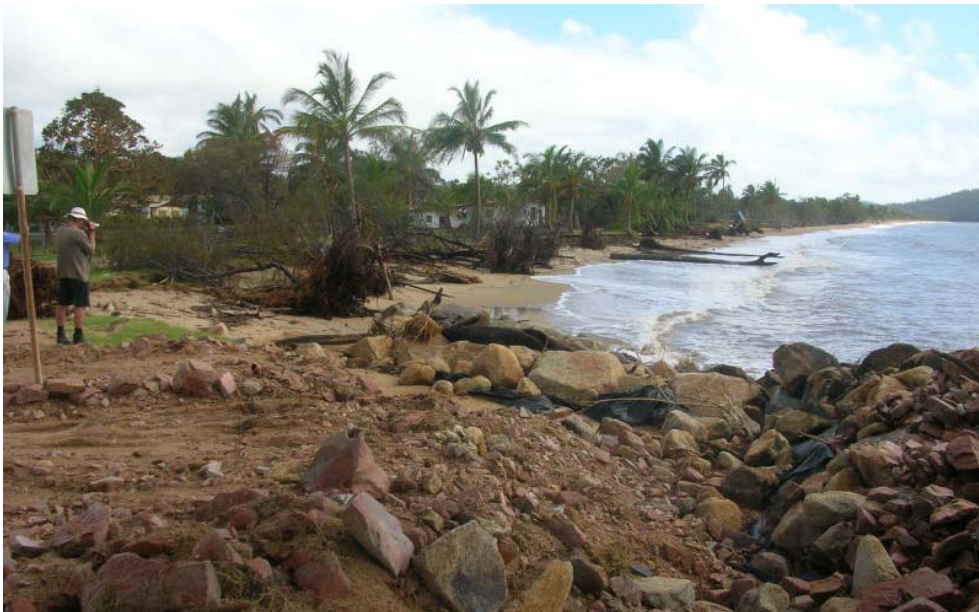
Photo 44. Slumping of the rock wall at Tully heads, exposing the underlying geotextile layer.
