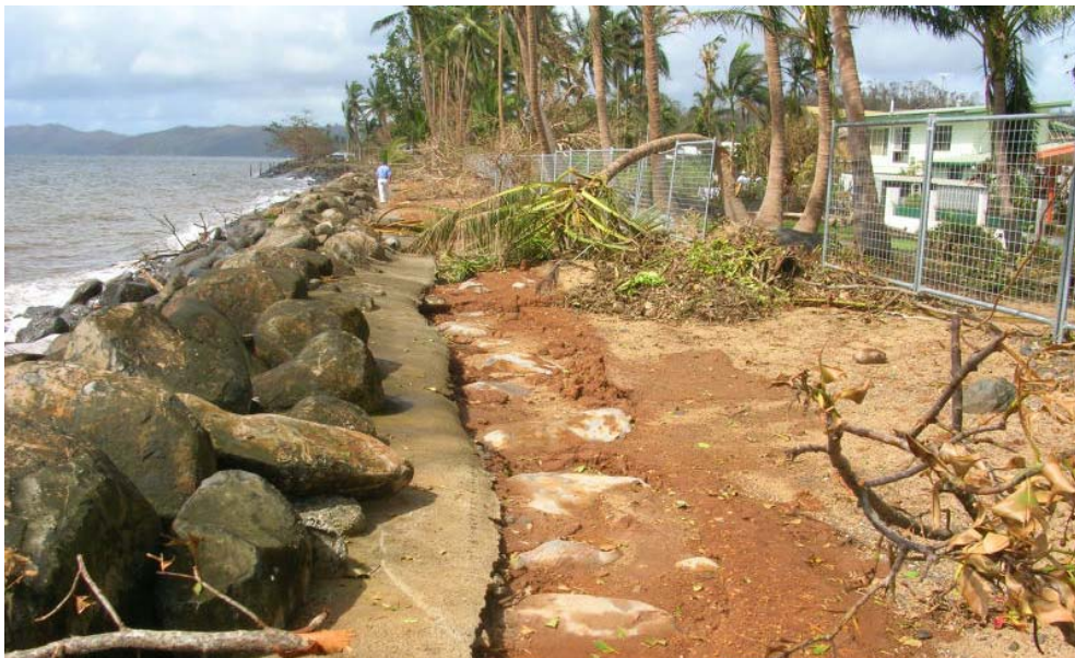
Photo 5. Undermining of rock wall at Flying Fish Point.
