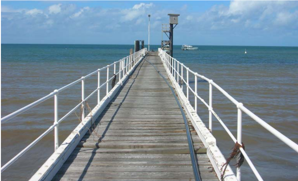
Photo 28. Clump Point jetty and storm tide gauge showing lifted timber decking and seaweed on the railing as a result of wave action.
