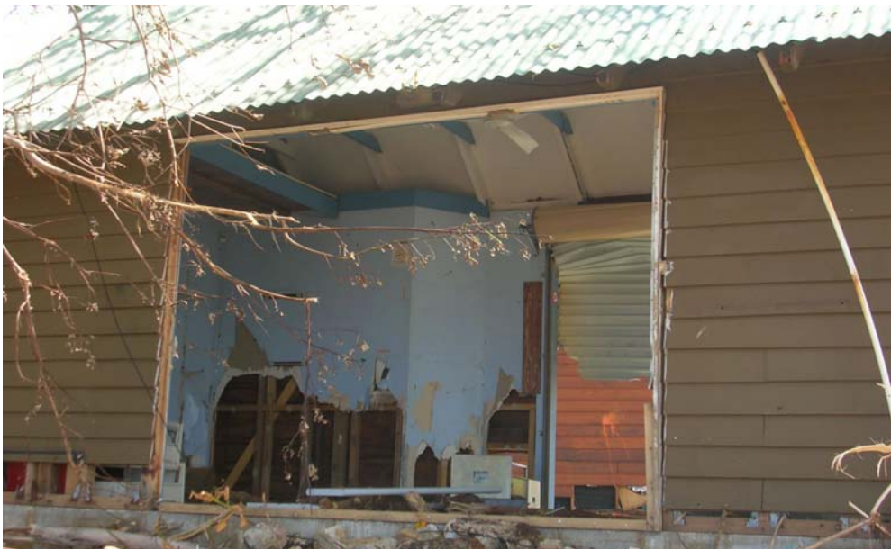
Photo 30. View of the interior damage to the building at Clump Point (picture taken from the ocean side of the building).
