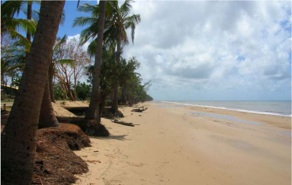
Photo 40. Erosion scarps at South Mission beach. Beach sand that had washed over the esplanade, had been piled between the palms.
