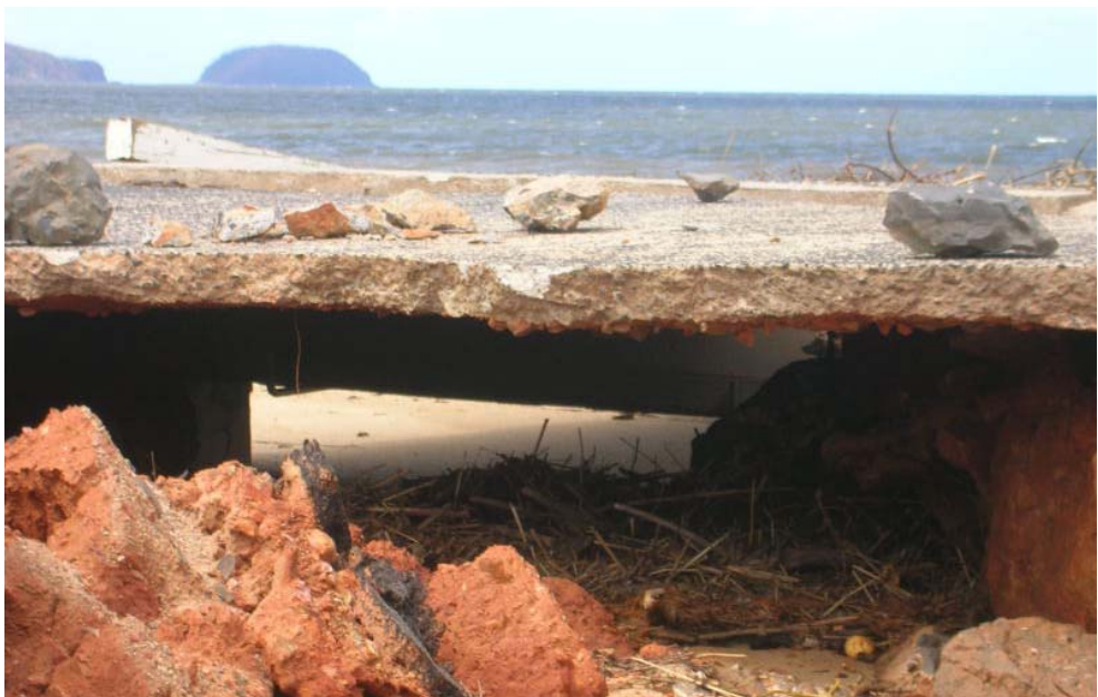
Photo 12. Eroded access road to the boat ramp at Cowley beach, undermined by wave action
