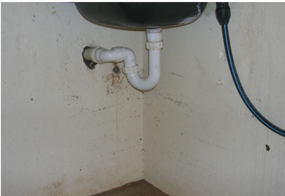
Photo 39. Inundation water levels within the public toilet block at South Mission beach.
