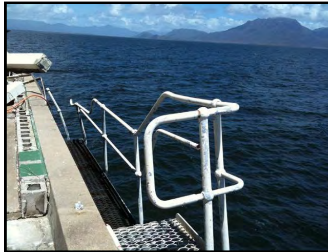
Photograph 33: DSITIA's offshore storm tide gauge at Lucinda - destroyed by TC Yasi (Source: DSITIA)
