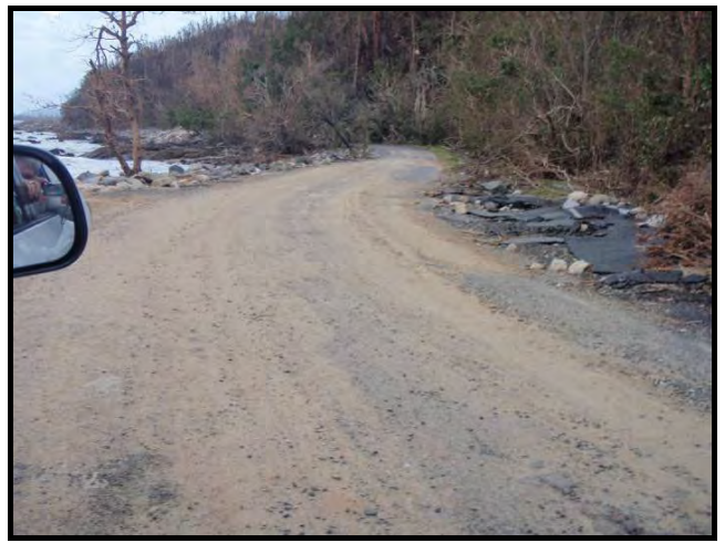
Photograph 11: Damage to road caused by TC Yasi between Clump Point and Bingil Bay (Source: DSITIA)
