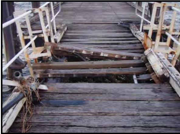
Photograph 14: Damage to Clump Point jetty during TC Yasi (Source: DSITIA)
