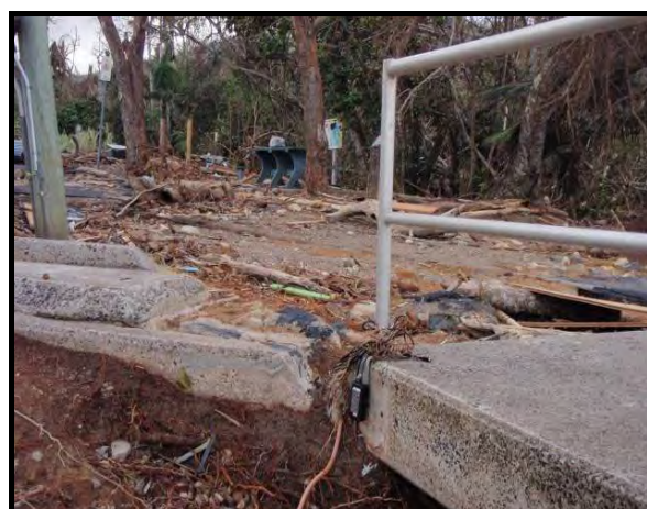
Photograph 13: Damage to Clump Point jetty (Source: DSITIA)
