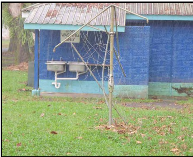
Photograph 5: Minor damage - Caravan Park toilet block at Bramston Beach (Source: DSITIA)
