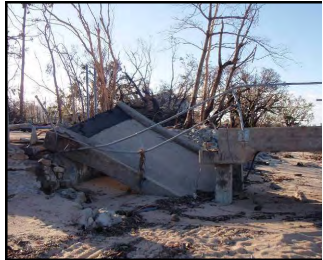
Photograph 29: Jetty damaged by TC Yasi at Cardwell (Source: DSITIA)
