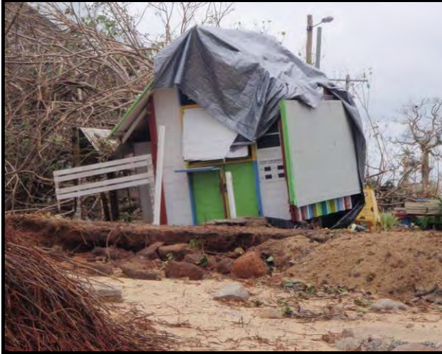
Photograph 18: Building damage caused by TC Yasi at Mission Beach (Source: DSITIA)
