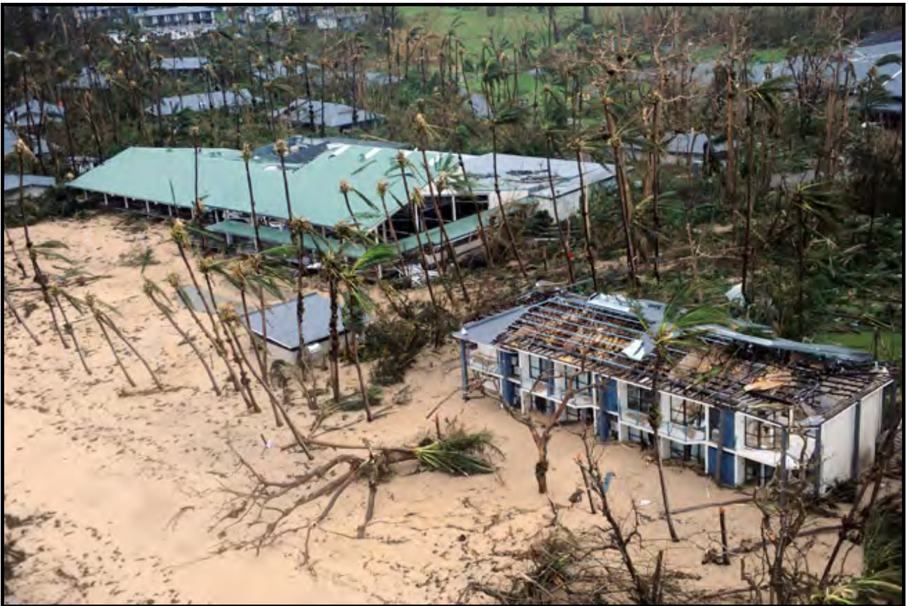
Photograph 45: Damage and mass sand deposition at Dunk Island Resort caused by the several metre storm surge during TC Yasi (Source: News Limited).
