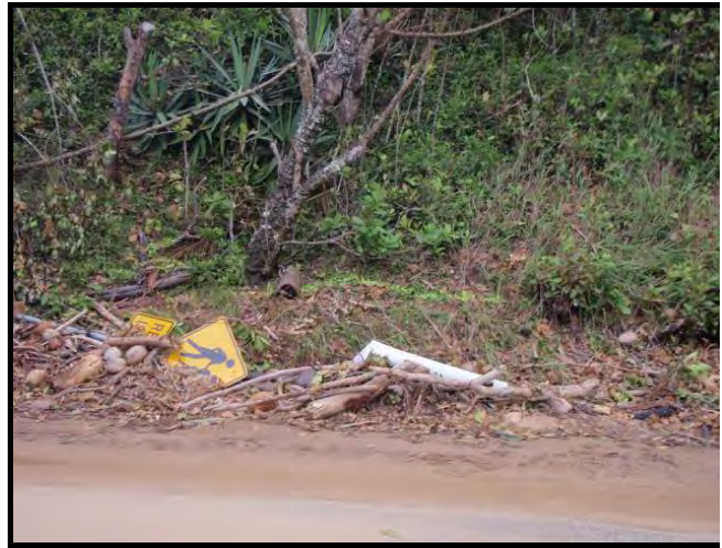
Photograph 9: Damage to road caused by TC Yasi between Clump Point and Bingil Bay (Source: DSITIA)
