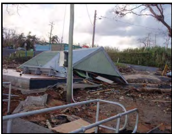
Photograph 12: Building and infrastructure damage caused by TC Yasi at Clump Point (Source: DSITIA)
