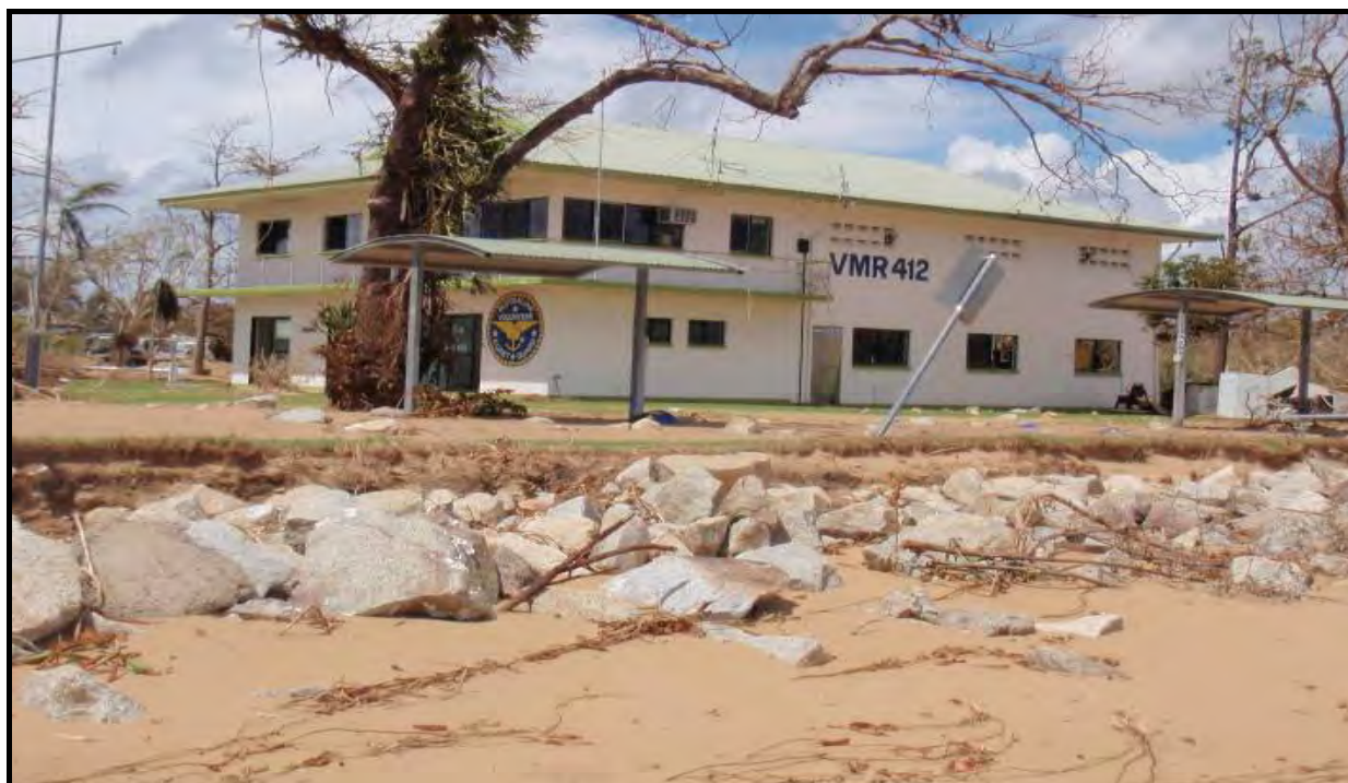
Photograph 21: Damage to Coast Guard building caused by TC Yasi at Hull Heads (Source: DSITIA)
