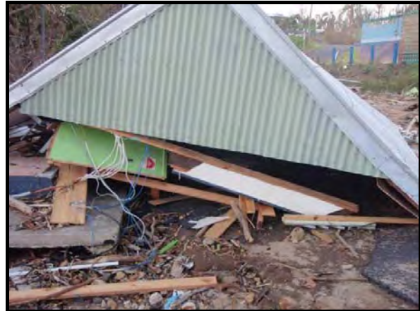
Photograph 15: Building damage caused by TC Yasi at Clump Point (Source: DSITIA)
