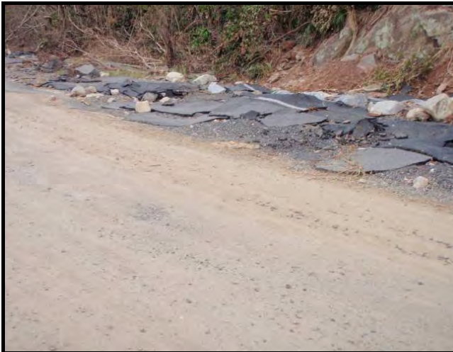
Photograph 8: Damage to road caused by TC Yasi between Clump Point and Bingil Bay (Source: DSITIA)
