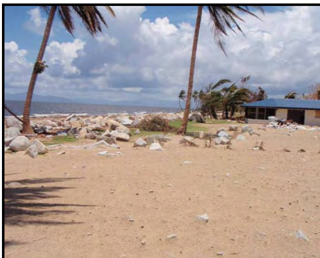
Photograph 26: Sand intrusion and rock retaining wall destroyed by TC Yasi at Tully Heads (Source: DSITIA)
