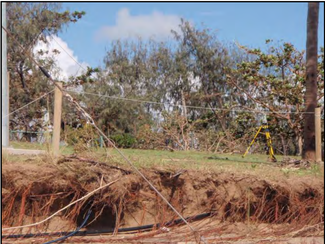
Photograph 37: Dune erosion caused by increased wave action during TC Yasi at Balgal Beach (Source: DSITIA)
