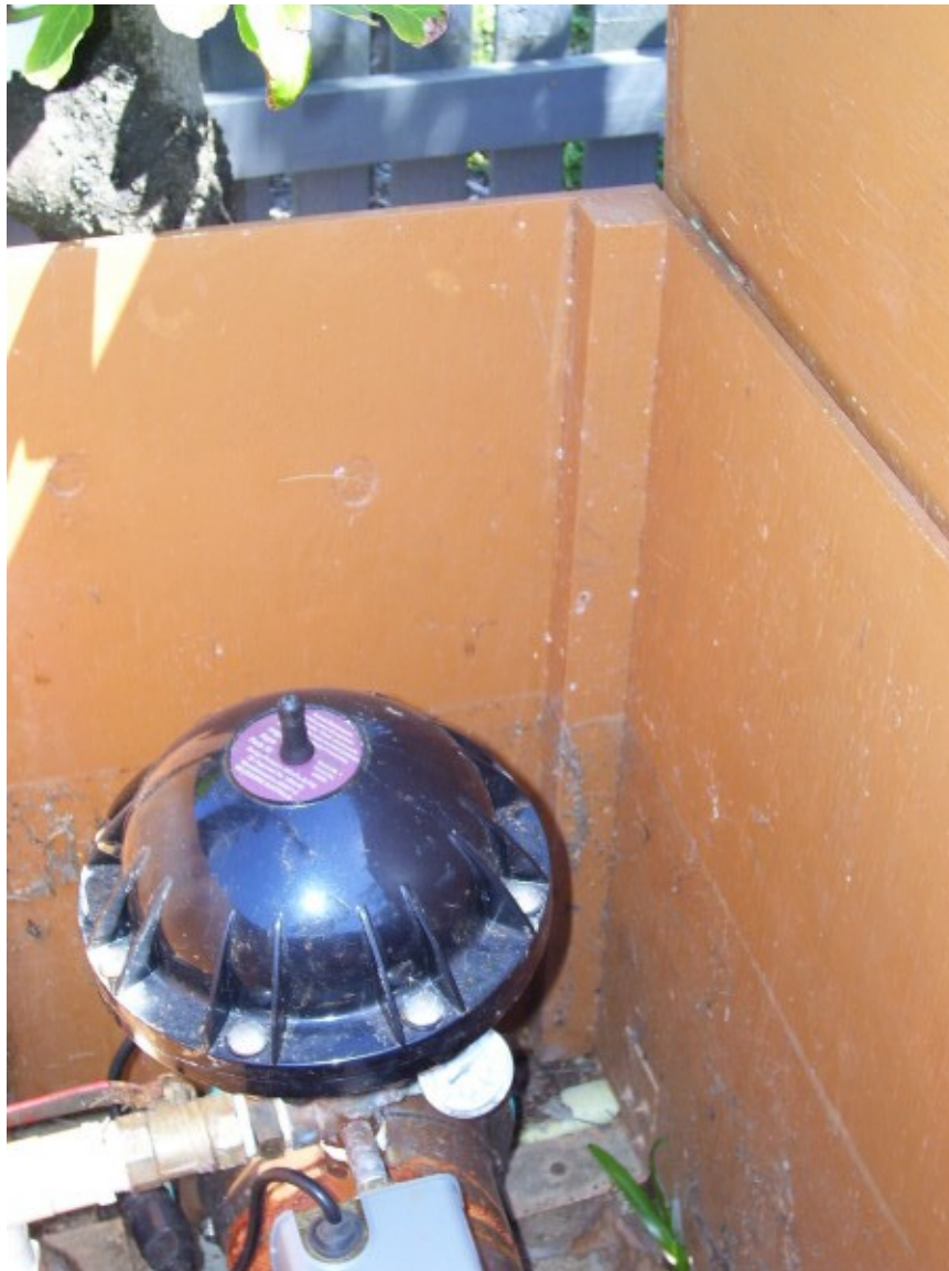
Water line in pump box in back yard, opposite the caravan park on Bambrook Avenue
