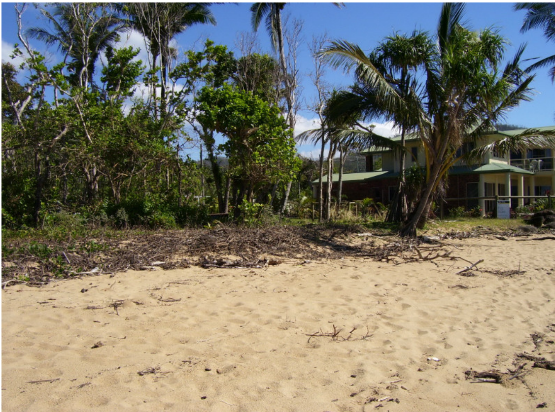
Looking towards the northwest from Beach Access 3, an erosion scarp of approximately 0.5m is evident, as is the debris
