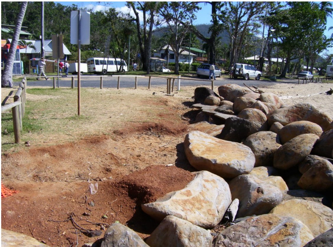
Erosion behind the rockwall outside the toilet block and the southern end of Flying Fish Point
