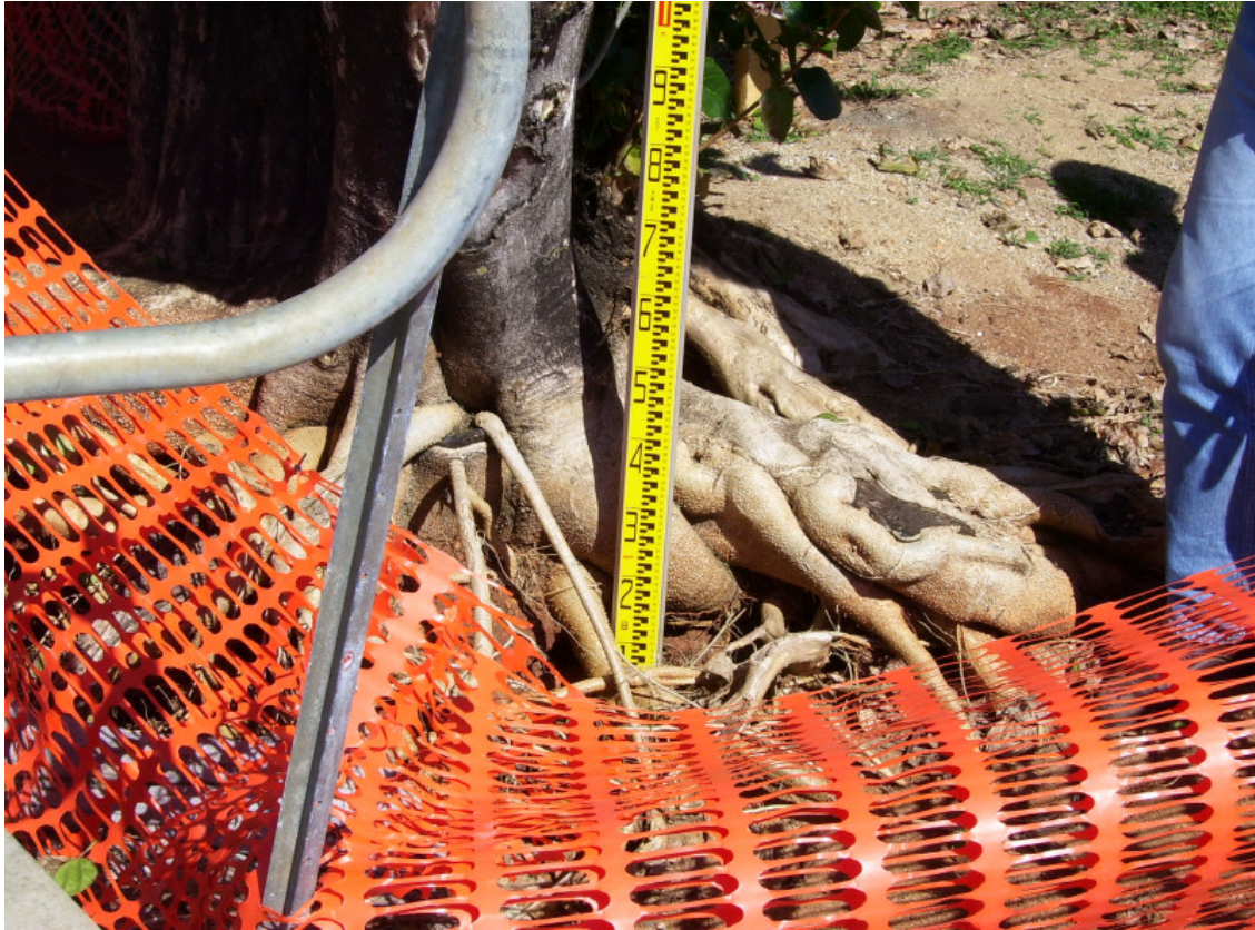
Tree outside the toilet block, where a scour mark was surveyed in March, it is evident that erosion has occurred around the roots of the tree
