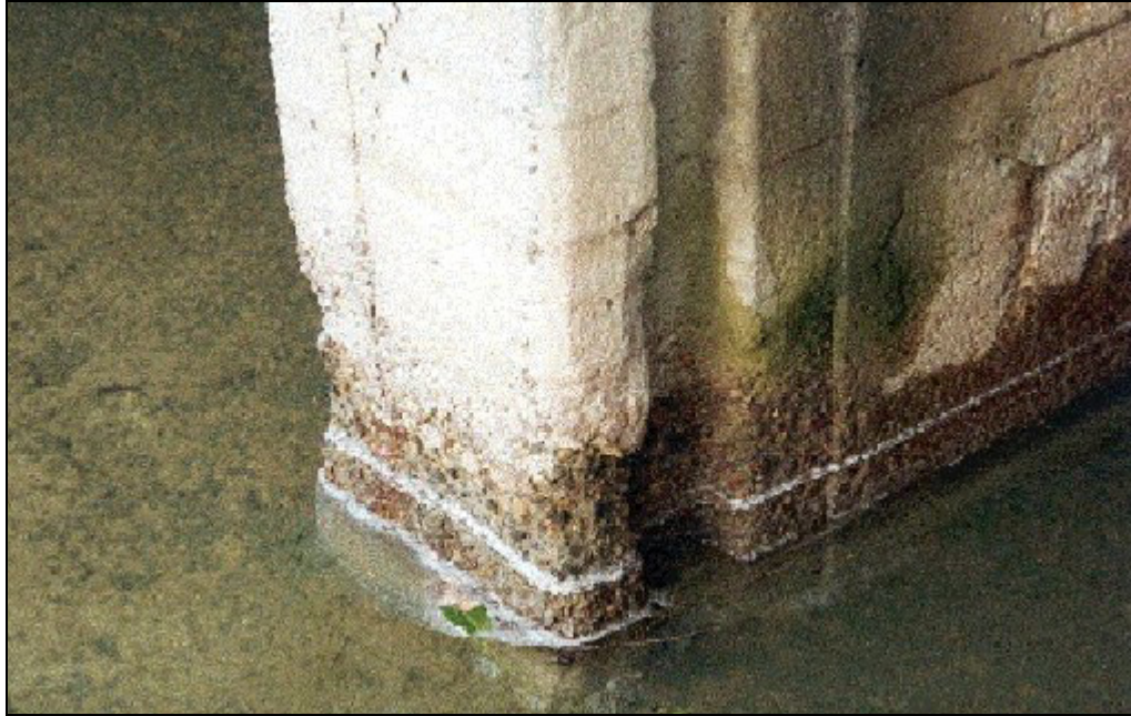
Plate 3. Acidified water from disturbed acid sulfate soils attacks concrete bridge pylons
