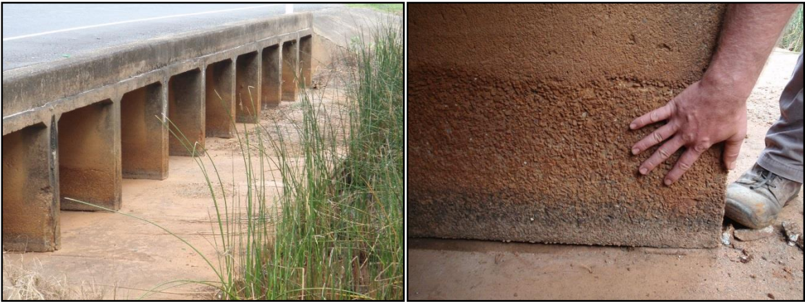
Plate 13. (a) Yorkeys Knob Road culvert (b) Acid water has corroded concrete of culvert
