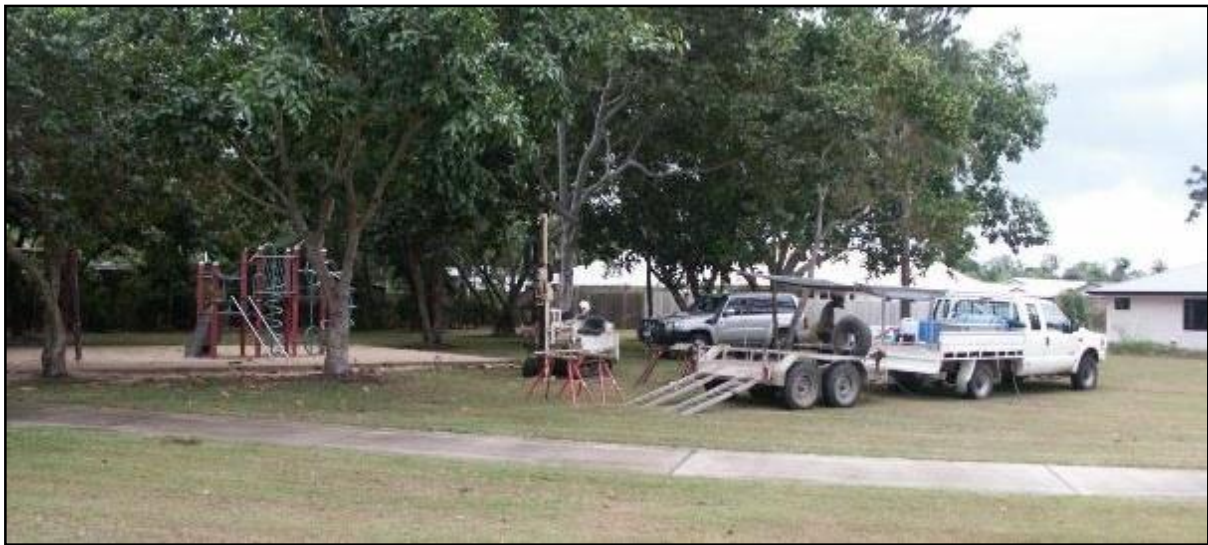
Plate 6. Site 224, Location: Hailing Park, Yorkeys Knob, Map unit: S5+, LiDAR elevation: 4.8m AHD, PASS depth: 5.05m, PASS elevation: -0.25m AHD.
