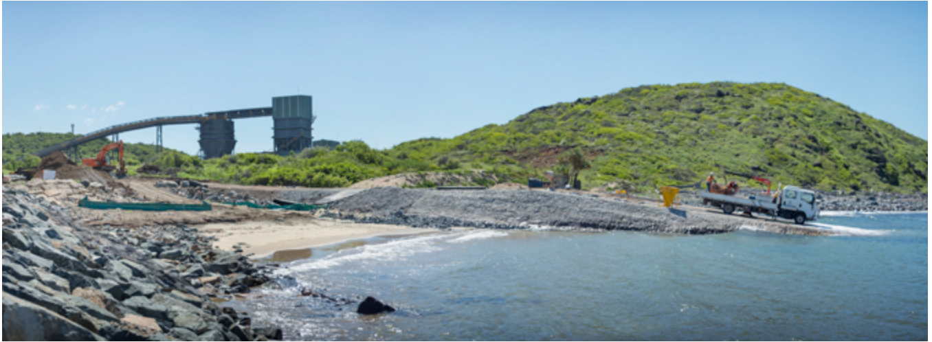
Material offloading facility under construction at the Port of Abbot Point. Source: NQBP
