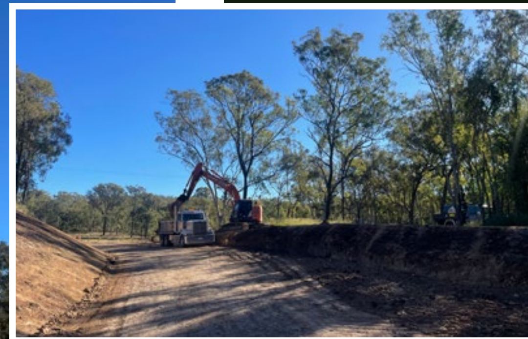
◀ A pad foot roller undertaking earthworks on Maidenwell-Bunya Mountain Road, South Burnett Regional Council
