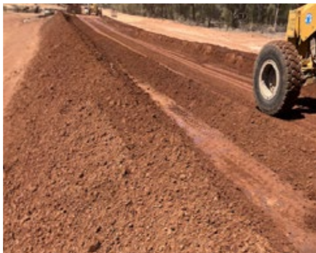
Jobs Gate Road, Paroo Shire Council - mixing of gravel prior to pavement
