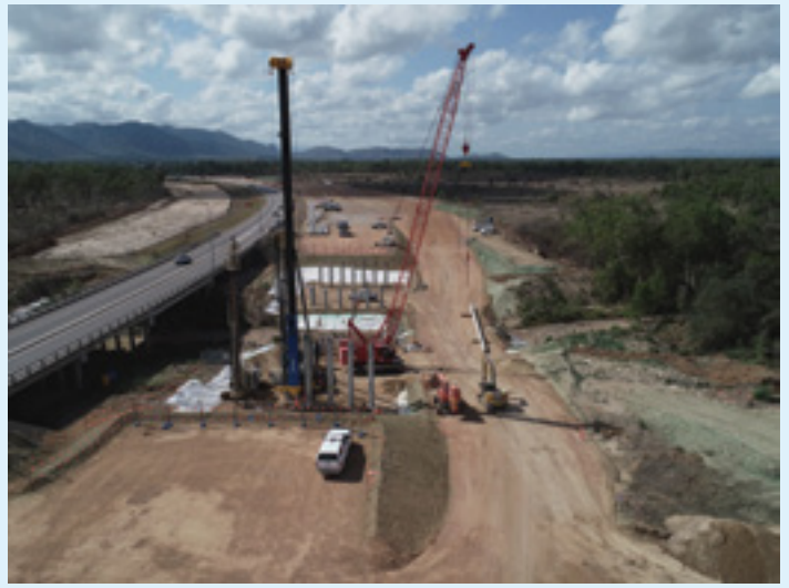
Townsville Ring Road Stage 5, Riverway Drive to Little Bohle River Bridge piling works (October 2021).
