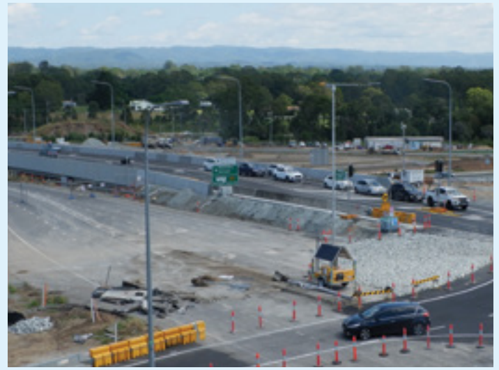
Bruce Highway Upgrade - Deception Bay Road Interchange, first new bridge opened to traffic (March 2022).
