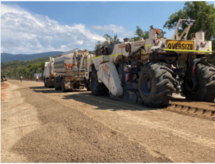
Townsville to Ingham, Hechts Road to Easter Creek Safety Upgrade (Project October 2021).
