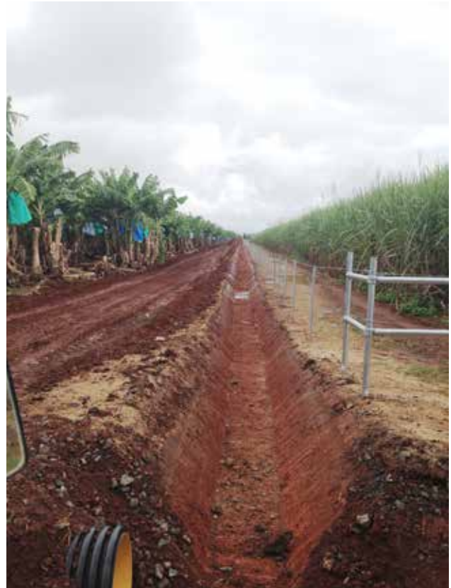
Figure 40: Drainage used to intercept water from neighbouring properties and divert water away from a production area
