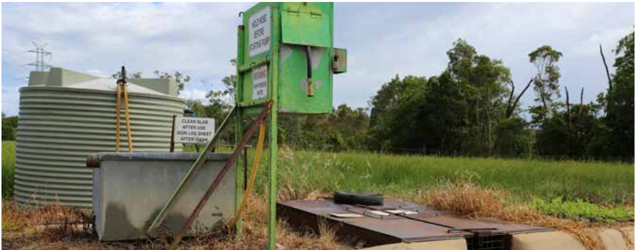
Figure 26: High-pressure hose and sump are essential elements of a wash-down facility
