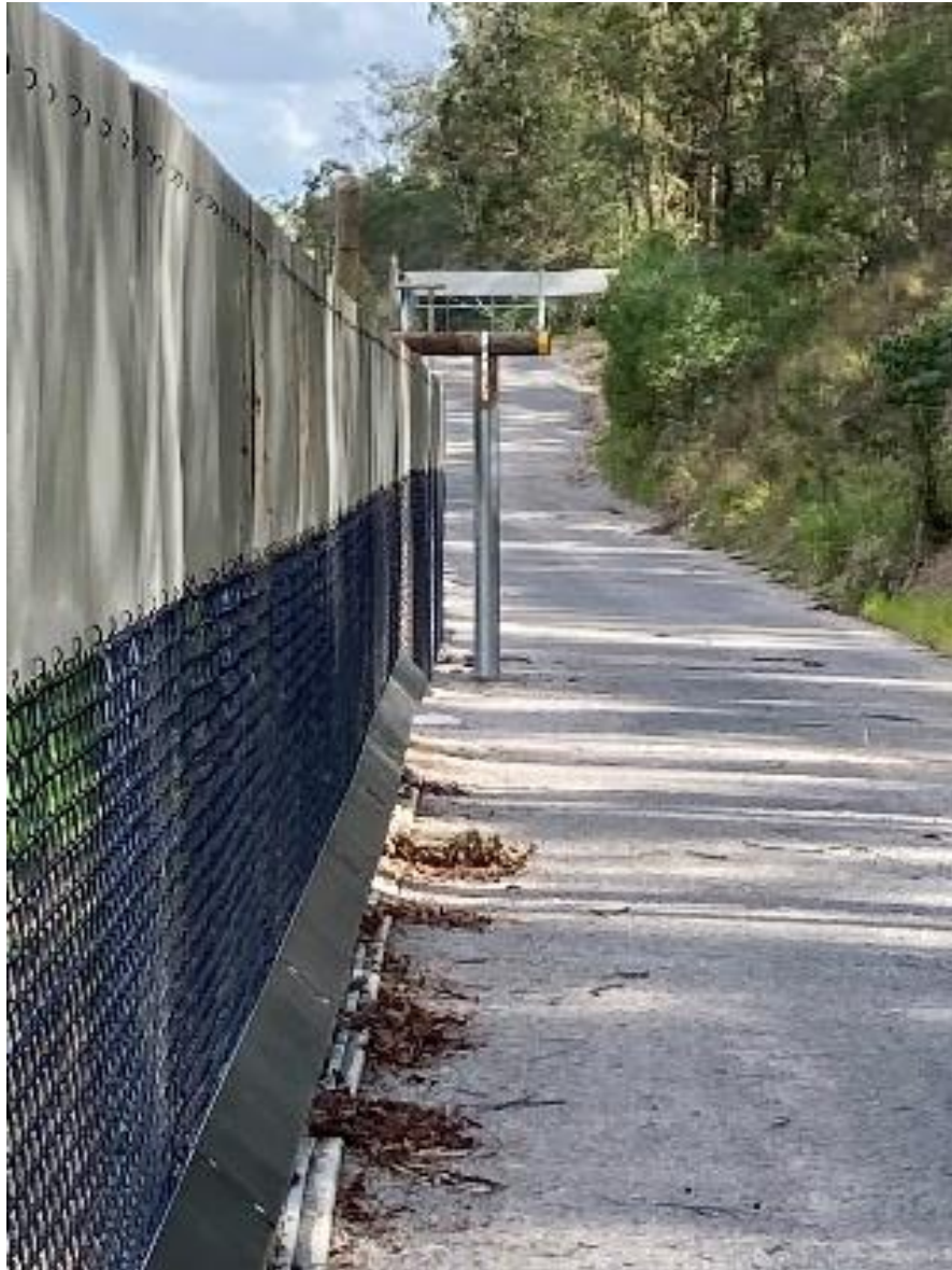
Figure 1. Permanent fauna fence with frog exclusion fencing and Koala escape pole adjacent to Bruce Highway
