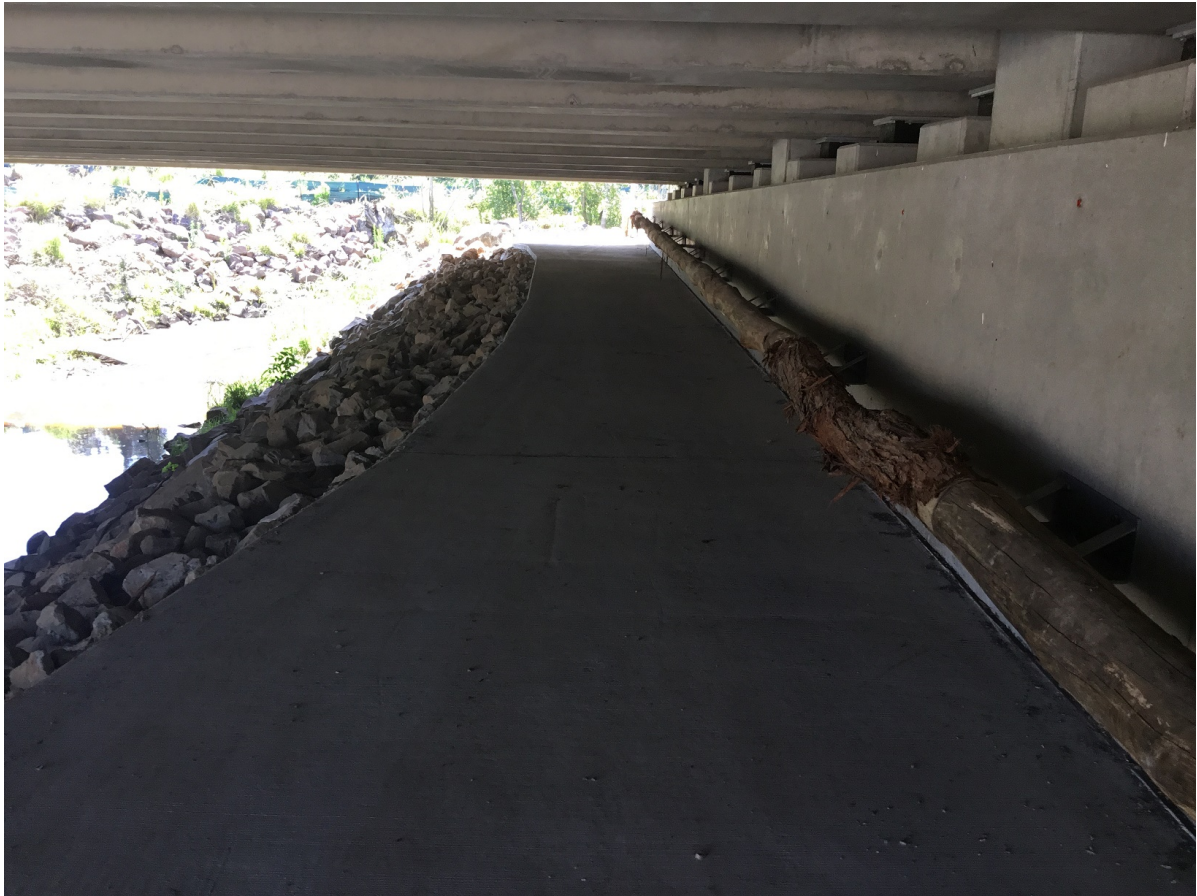
Figure 4. Fauna ledges installed under Mooloolah River bridge
