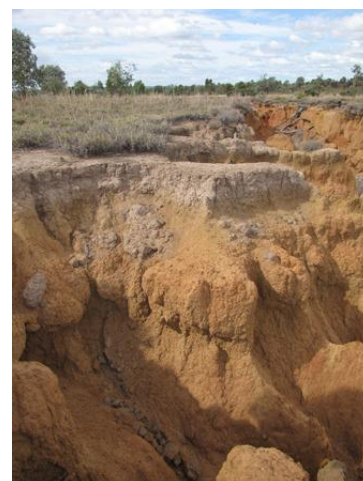
Figure 5. Photo of a stable soil overlying a dispersive subsoil
