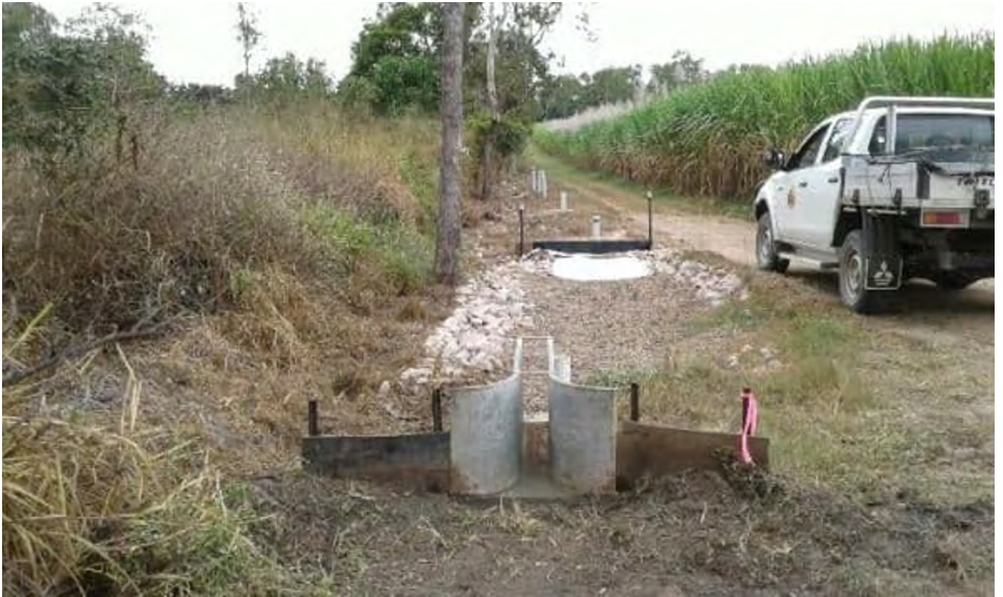
Figure 18: Flume installed on a sugarcane farm to monitor surface water discharge entering a treatment system.
