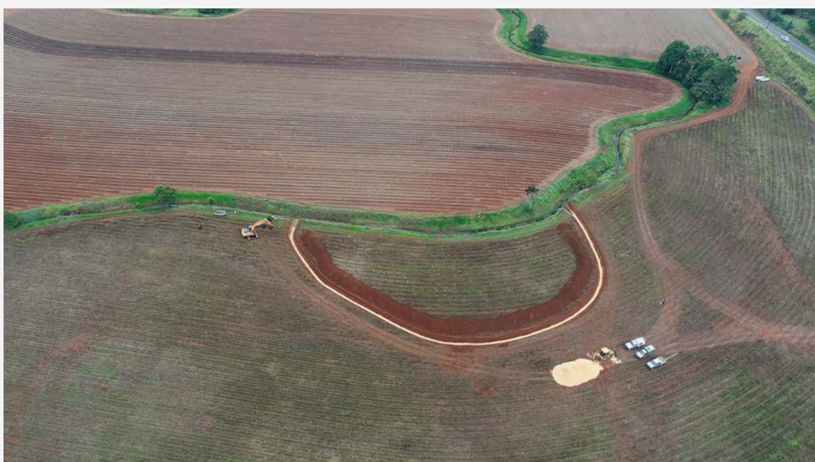
Figure 1 Aerial image of ag-pipe bioreactor under construction, showing cane crop and drainage line into which the bioreactor outlets. Source: WTMIP
