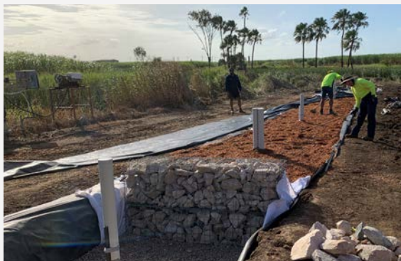
Figure 2 Bioreactor looking from the inlet toward the outlet, showing the rock gabion separating the inlet from the woodchip.
