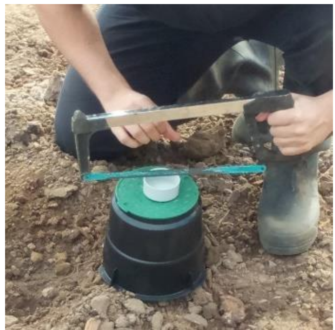
Figure 2: Cut four evenly spaced cuts on the 'wall' of the top cap to enable easy removal of the cap.
