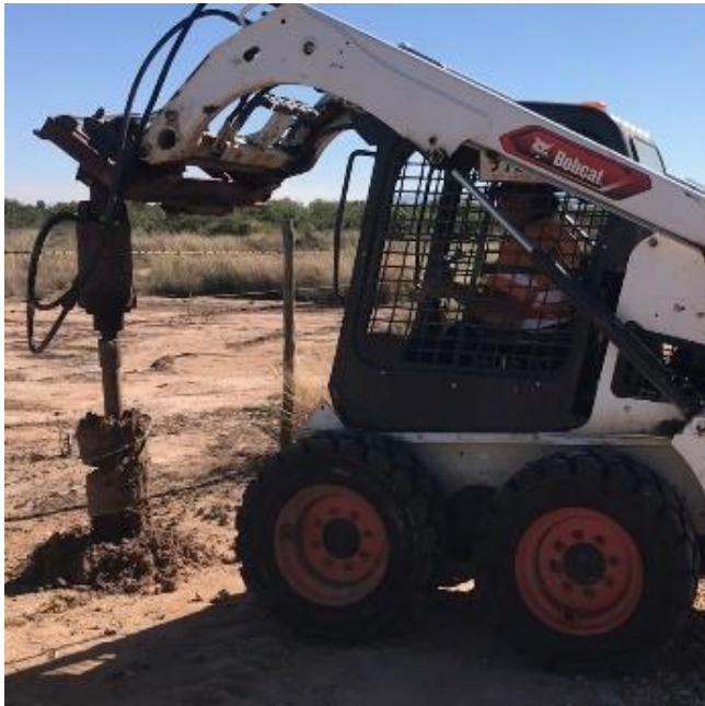
Figure 1: An auger and bobcat can be used to drill a hole quickly.
