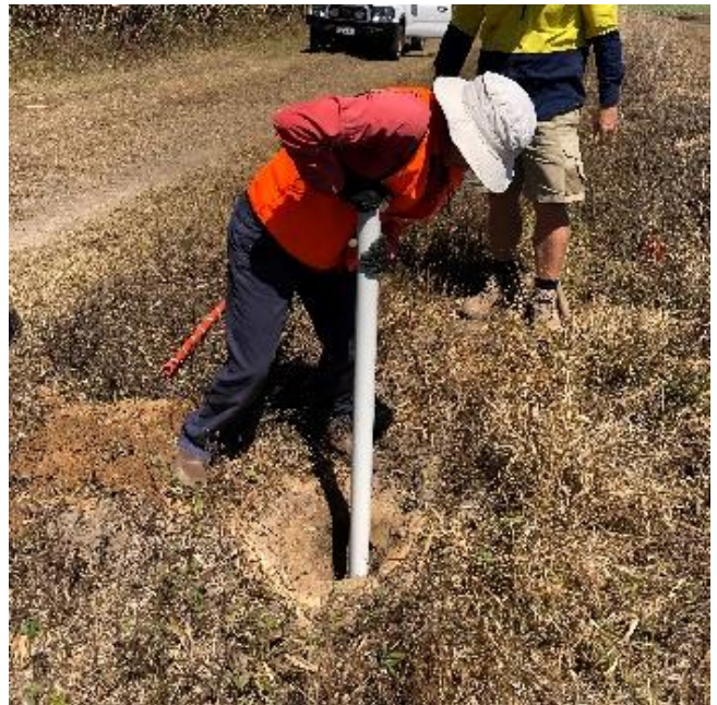
Figure 3: First, backfill the hole with fine gravel or coarse sand to 0.1-0.2m above the screen section of the piezometer.
