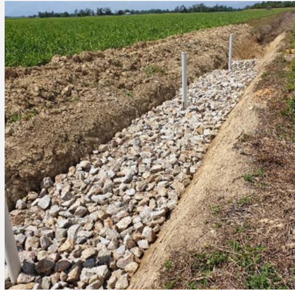
Figure 2 In-line bioreactor bed showing rock on top of woodchip zone for stability.
