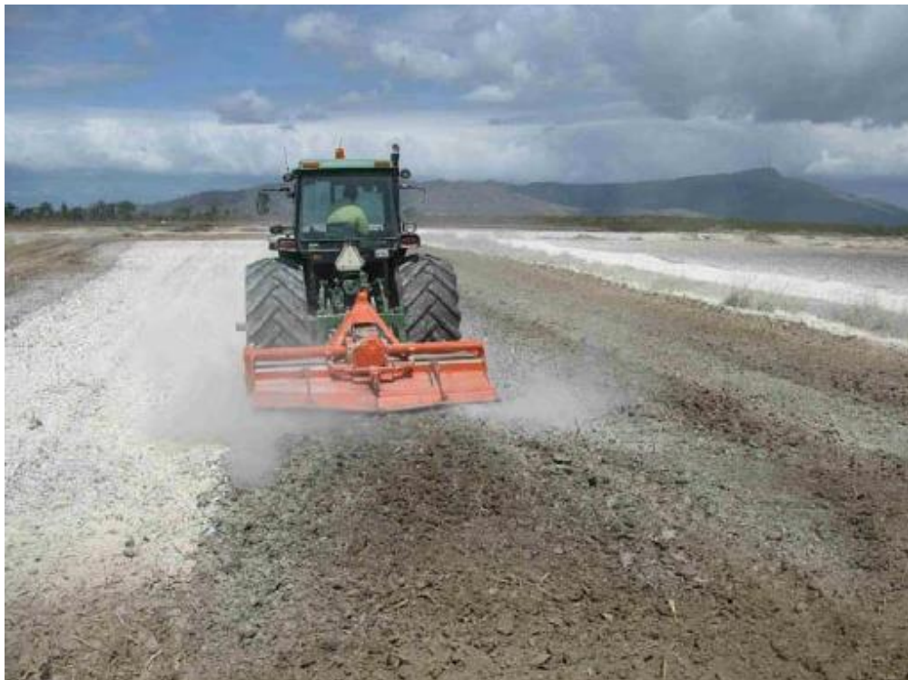
Figure A63-2: Rotary hoe mixing in surface applied aglime within excavated fill material
