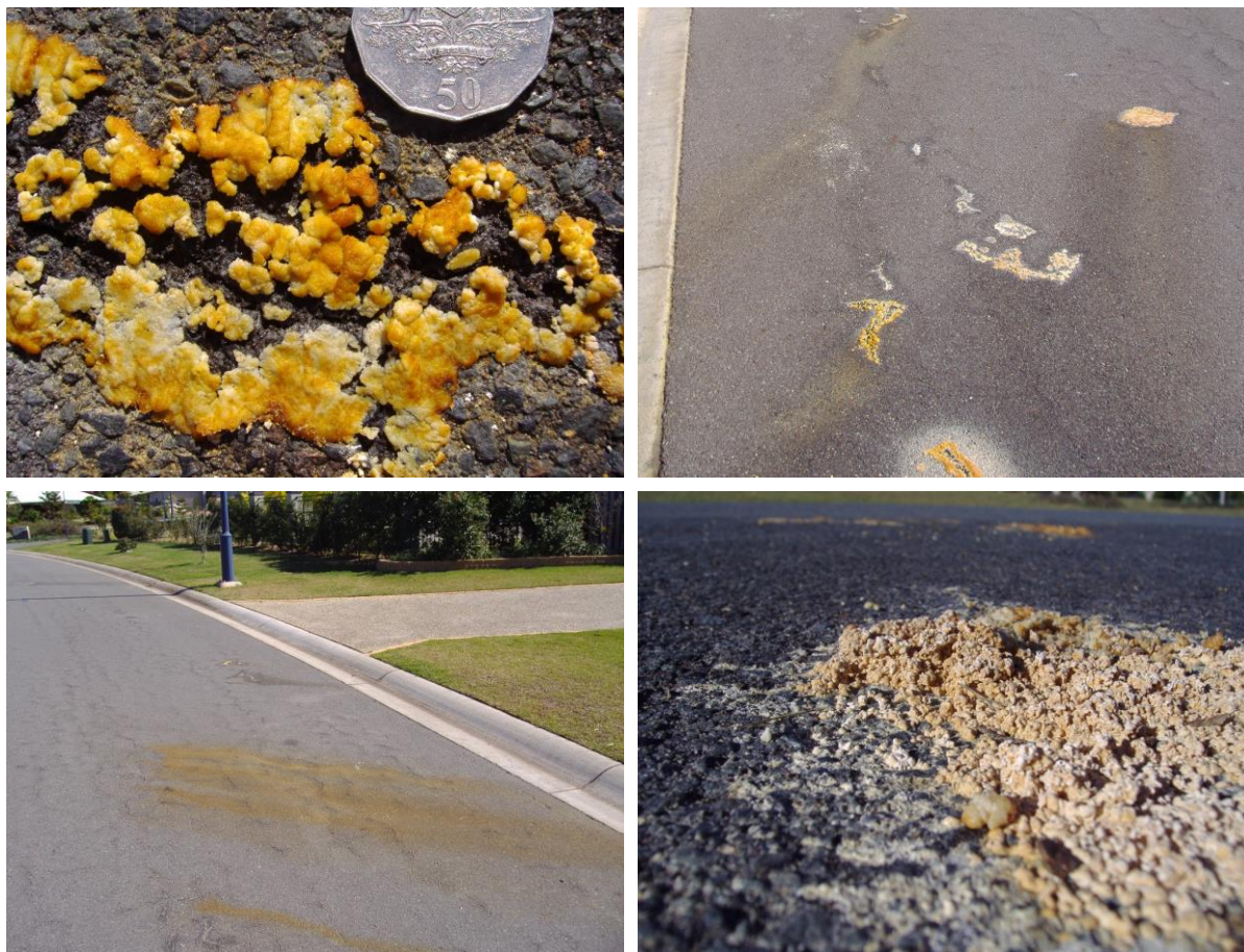
Figure 16: Acidic salts and minerals on asphalt surfaces
