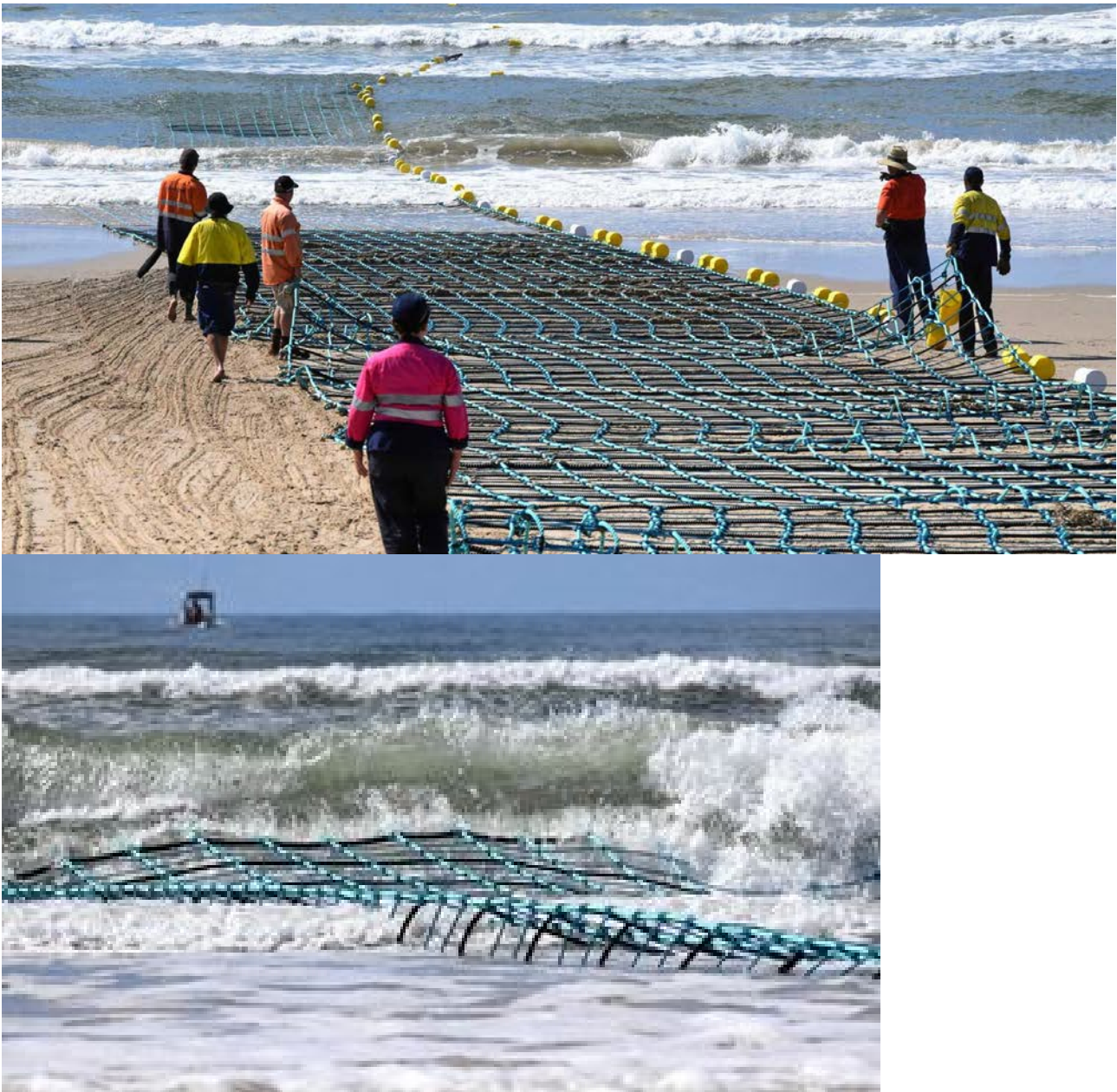
Figure D3 A bionic barrier being installed at Lennox Head and the aftermath during heavy weather
