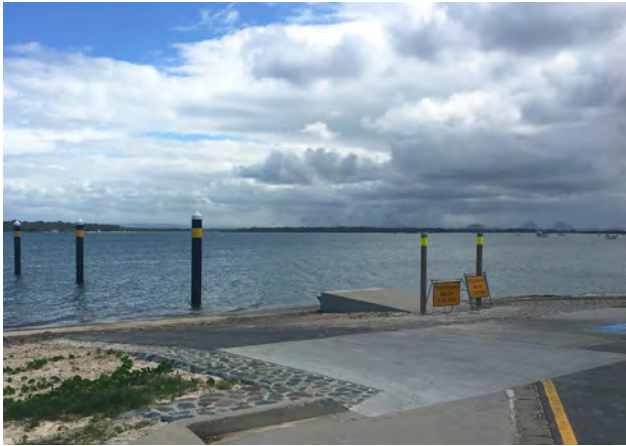
Maintenance dredging works were completed on the Bellara boat ramp at Bribie Island.
