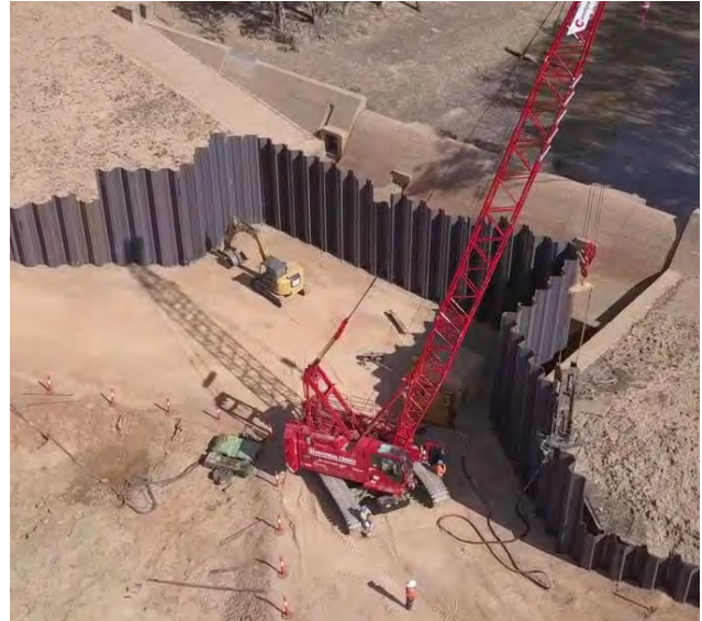
Aerial photo of the works to reinforce the Lloyd Jones Weir, south of Barcaldine.
