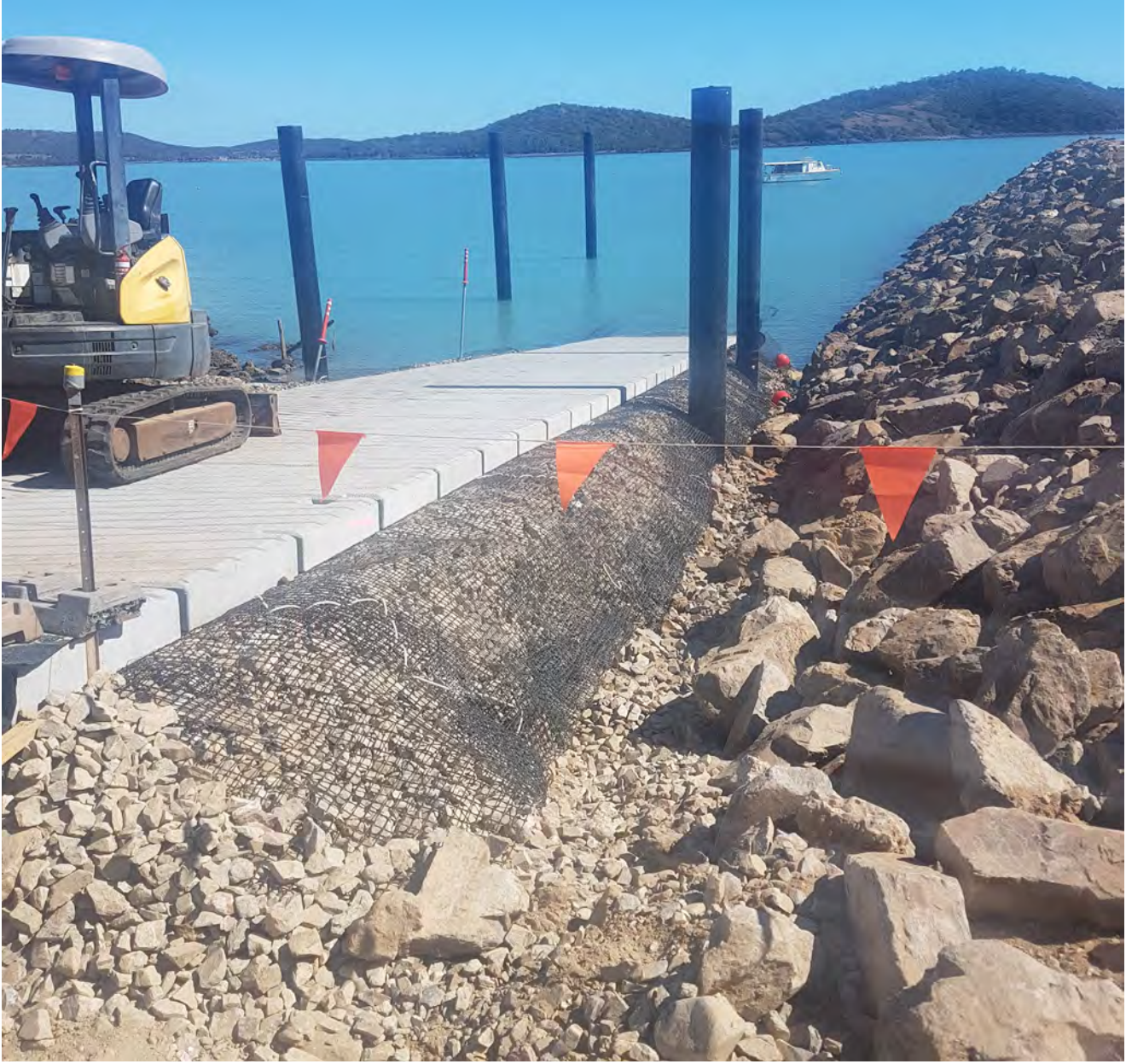
Crew commencing constructions works for the breakwater on the Stanage Bay boat ramp.
