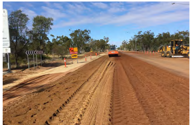
Works underway on the Landsborough Highway outside Barcaldine as part of the Barcaldine South Upgrade.
