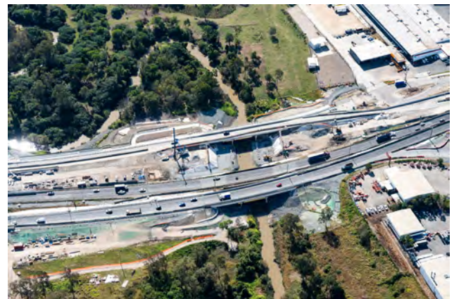
Ipswich Motorway Upgrade – Rocklea to Darra (Stage 1) project: Construction of new motorway bridges over Oxley Creek floodplain (Photo credit: R2D Aerials Press 39).
