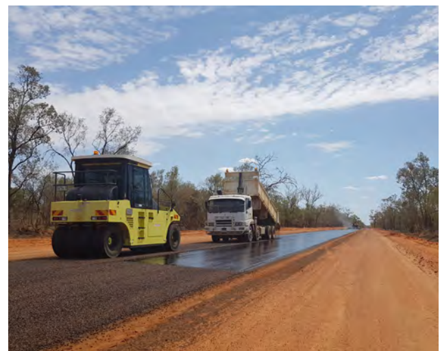
Works underway on Blackall-Jericho Road as part of the Western Roads Upgrade Supplement.
