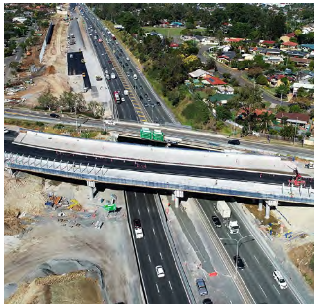
The first two lanes of the new Underwood Road four-lane bridge over the Pacific Motorway (M1) at Eight Mile Plains.
