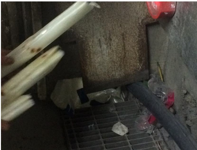
Figure 5: The 12 level crib room wash basin drainpipe
