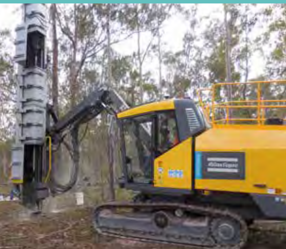
A percussion drill being used to sample the hard-rock resource to a depth of 25 metres; DAF staff provided assistance through site set-up, logistics and supporting field sampling activities
