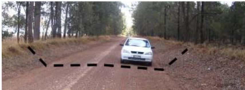
Figure 13 – Incorrect road maintenance can lead to subsurface roads from which runoff can't escape.
