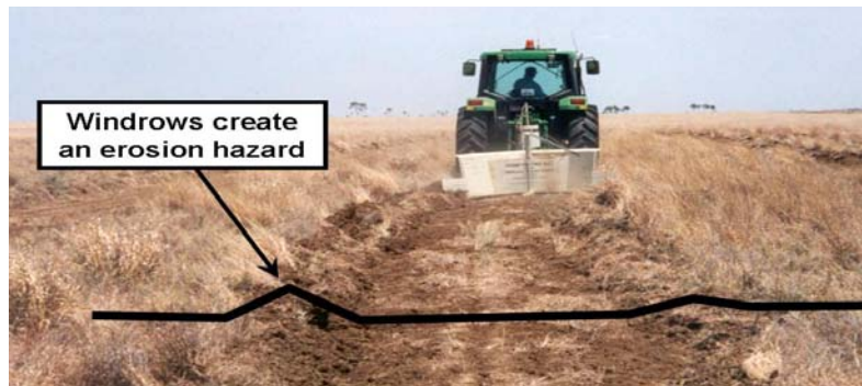
Figure 3 – Windrows created during firebreak construction may concentrate and divert runoff.
